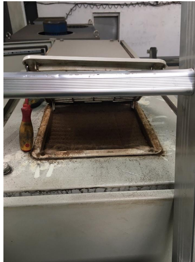
BLM Tube Laser – Clogged Filter
