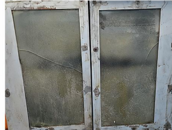
Damaged Front Doors
