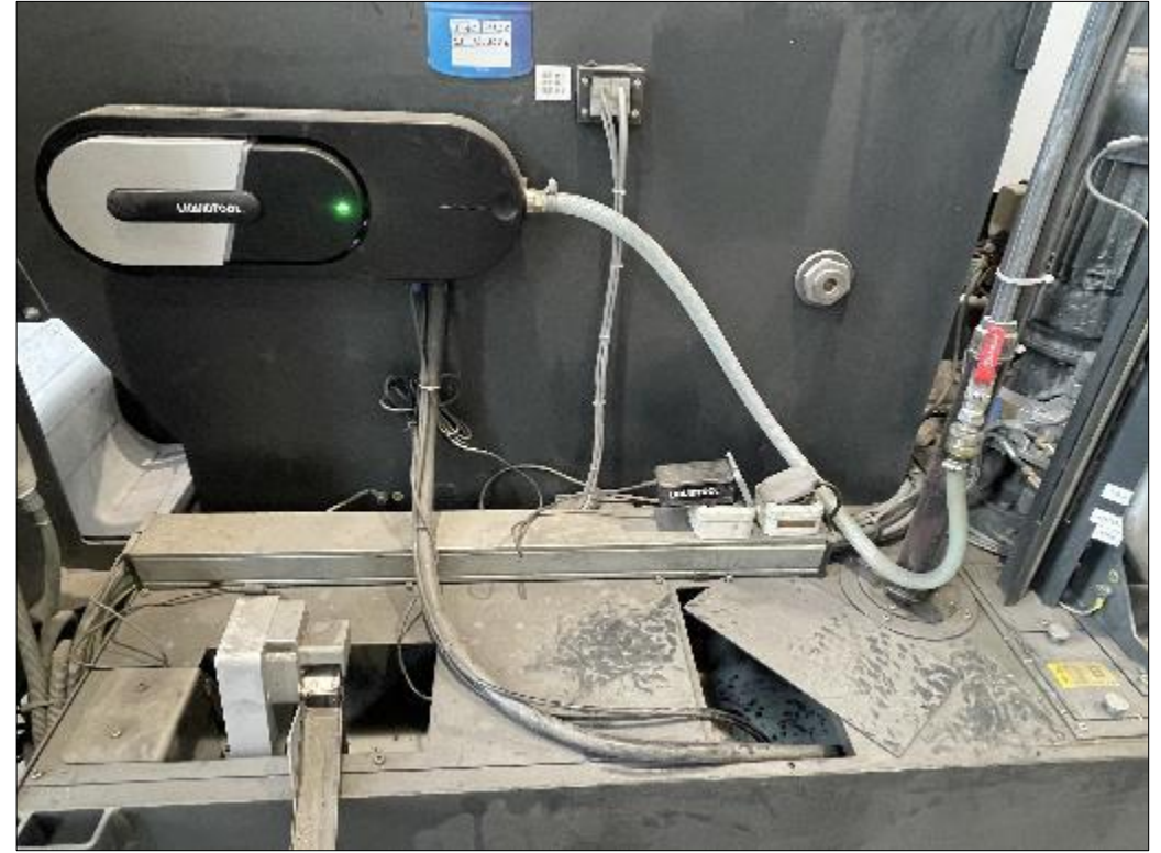
Covers Above the COT Tank with the Automatic Refill Sensor
