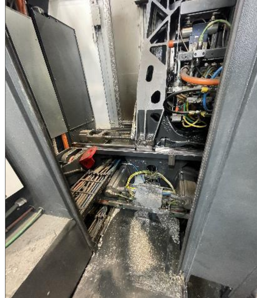
Chip Accumulation Behind the Machine Near the Moving Parts
