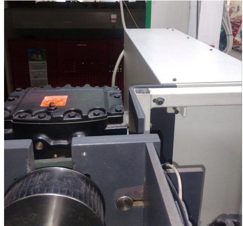
Bending machines – electric cabinet
