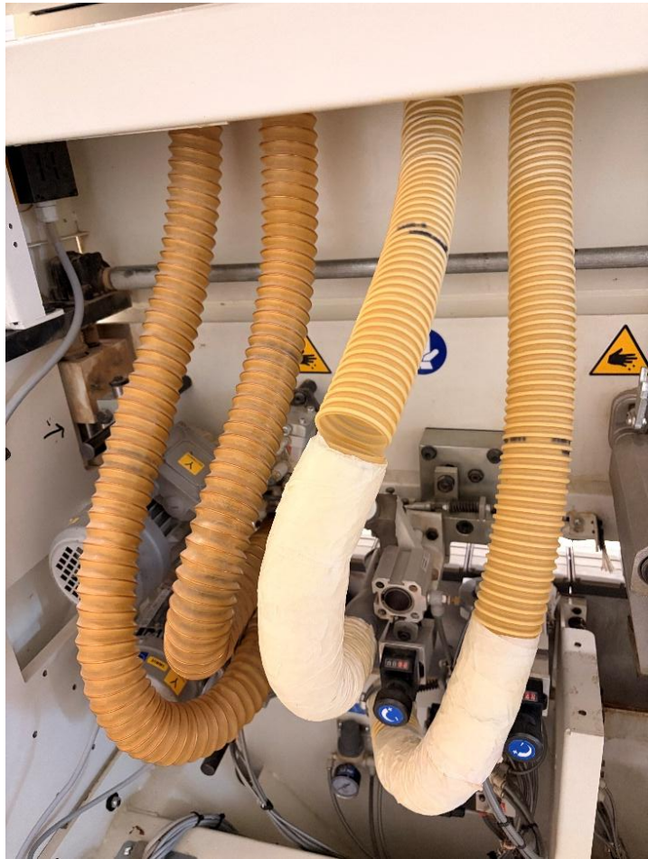
SMC edging machine broken pipes of duster system
