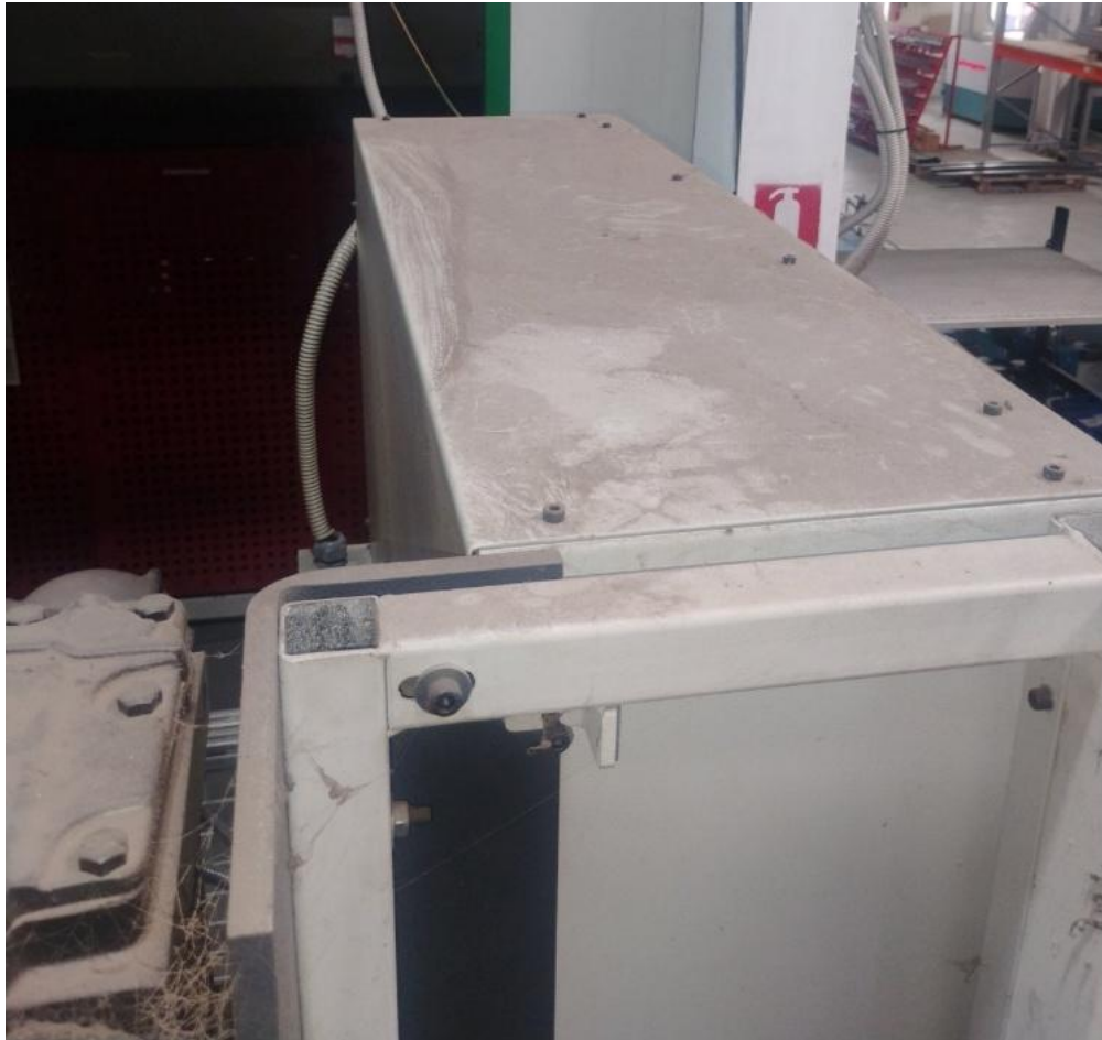
Bending machines – electric cabinet
