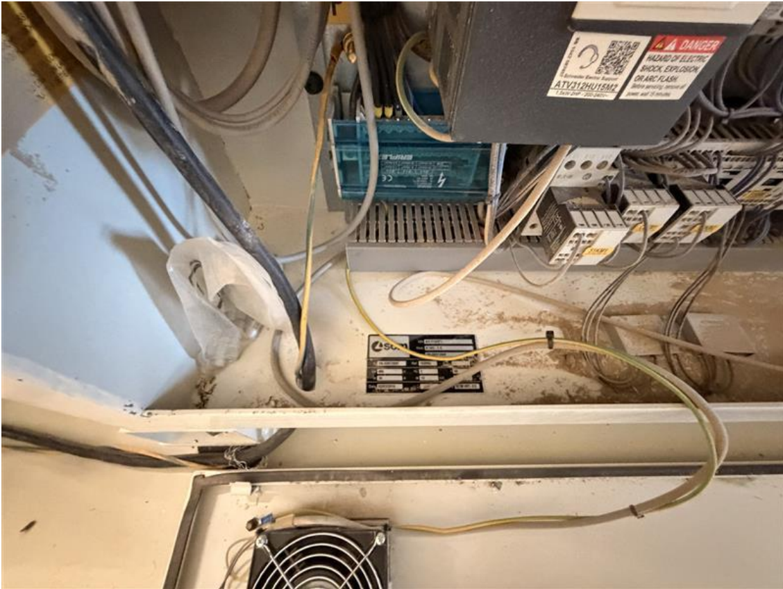
SMC edging machine Dirty electric cabinet
