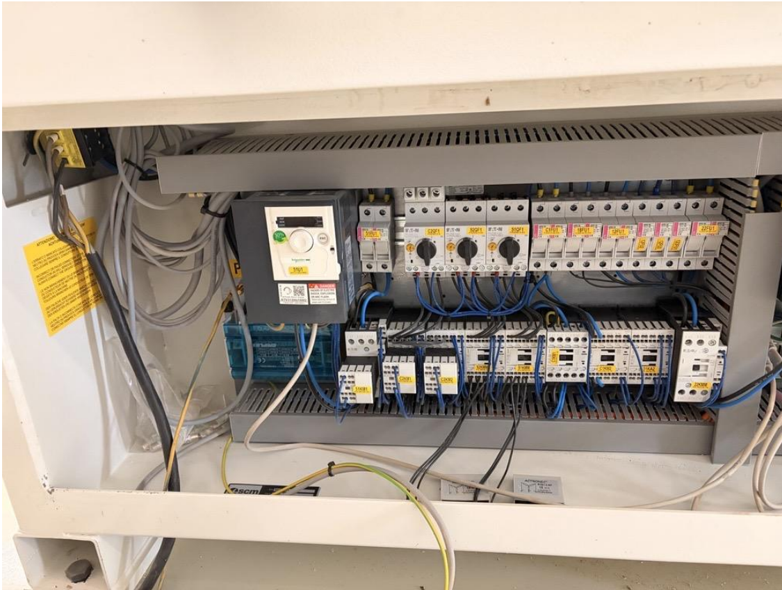
SMC edging machine Dirty electric cabinet
